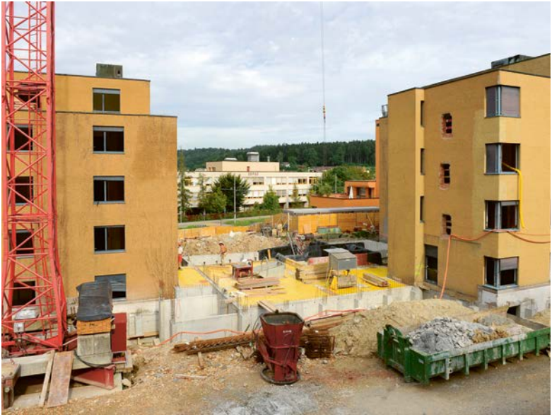
4.12 Renovation and extension of the two buildings at Kraftwerk 1's second project, Heizenholz, 2010
