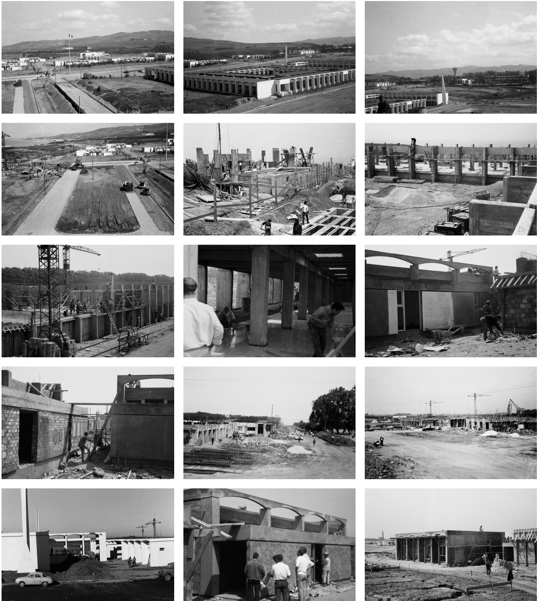
Figs. 62a-o The construction of the first phase of Rocher Noir, completed in 1961
